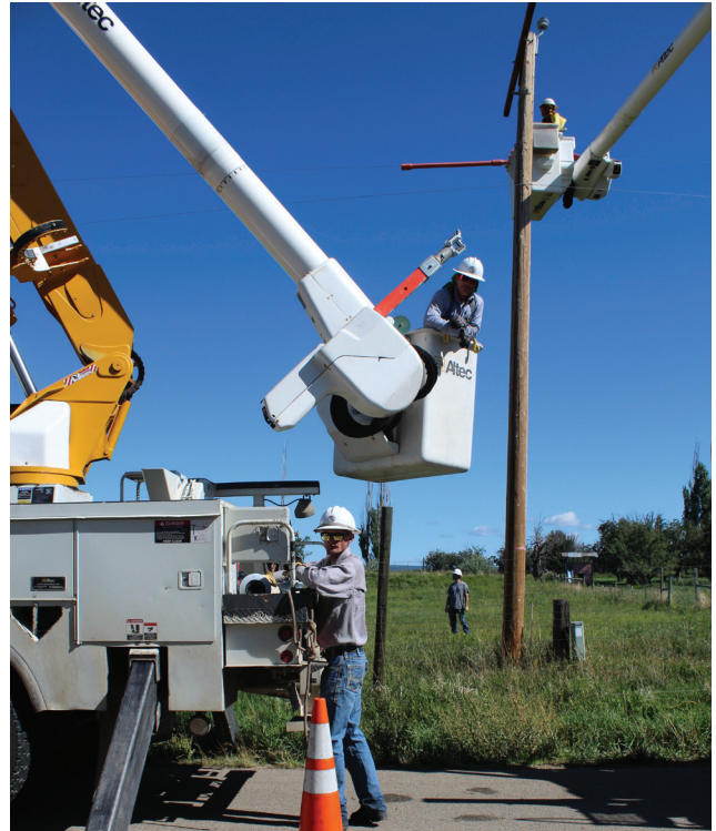
EEA Linemen Matt Ruggles, Shad Bellmire, Brett Crouse, and Chase Suckla work on the three phase upgrade to Weber Canyon serving members south of Mancos, Colorado. This project is part of EEA's construction work plan to increase capacity where we see consistent growth. Photo by Denise Moore
