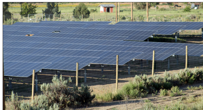
▲ Totten Lake solar generation station located northeast of Cortez is one of three local renewable generators that delivers clean energy to EEA members.
